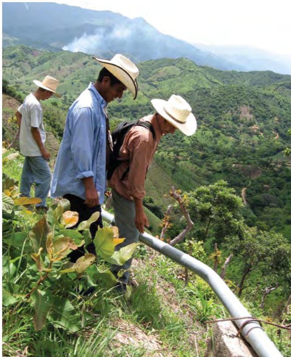
Felipe, Ganuario and Jose, members of the water committee in Gualcea, Honduras, check on the water distribution line that runs from the tank to the community of Gualcea.
