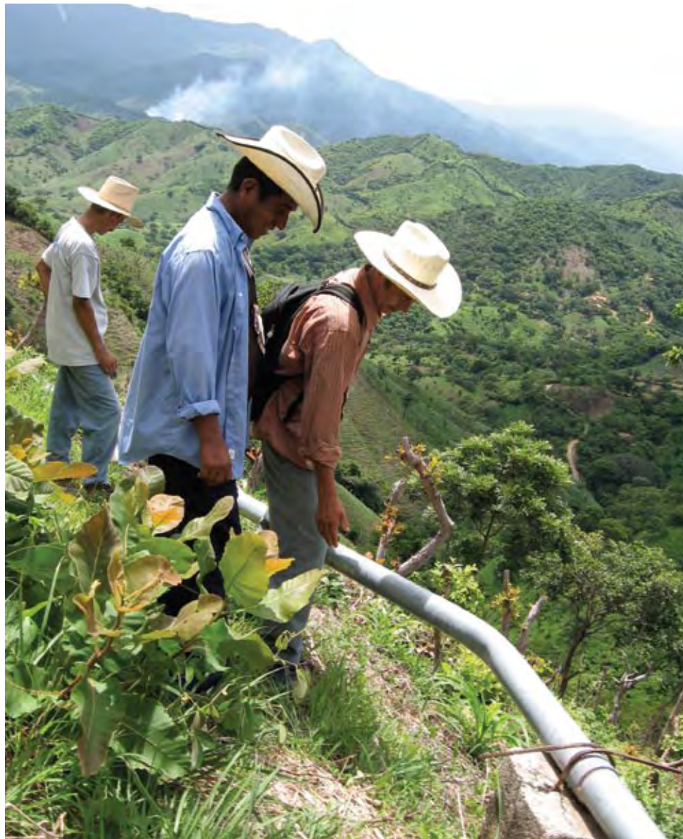
Felipe, Ganuario and Jose, members of the water committee in Gualcea, Honduras, check on the water distribution line that runs from the tank to the community of Gualcea.
